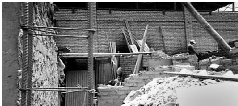
Construction site with crumbling chrysotile asbestos in Peru - Courtesy CAW
